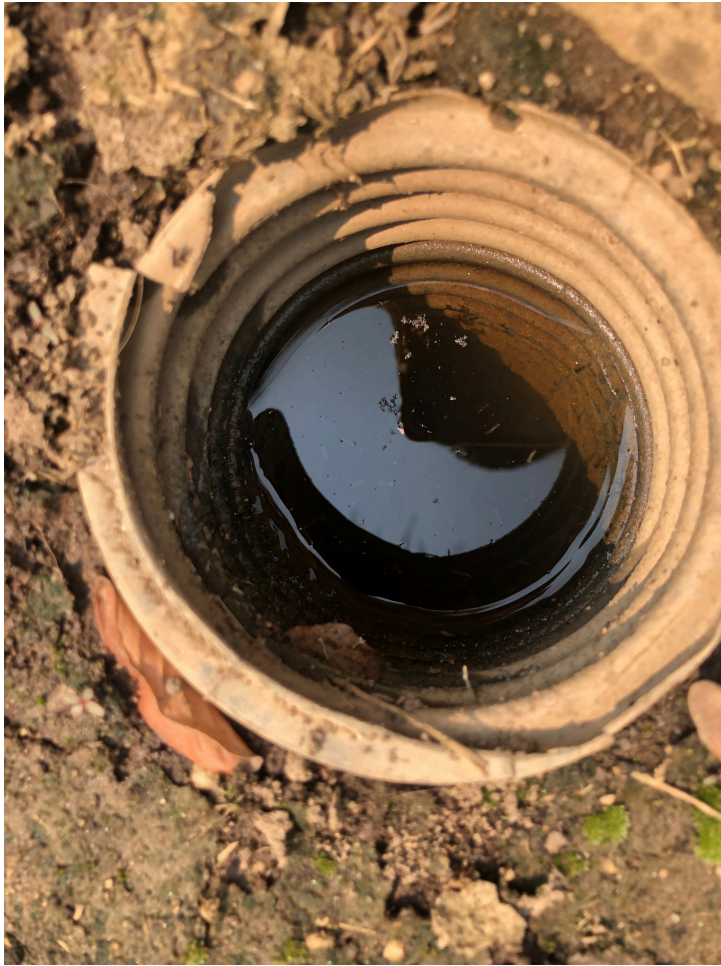
Yard drains that are not properly screened and capped are among the most frequently identified sources during service requests.
