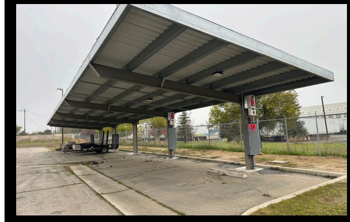
Solar covered parking at the Parlier (above) and Clovis (below) offices.
