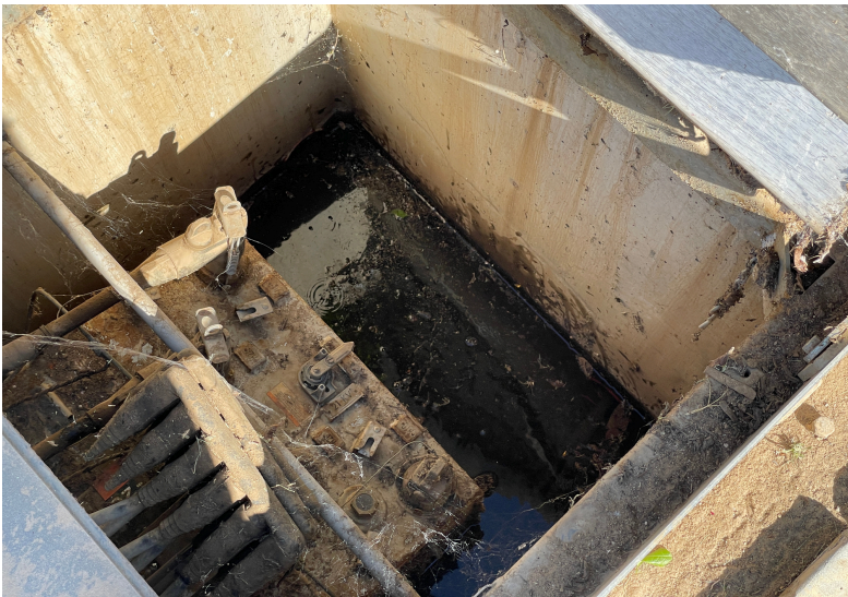
A utility enclosure requiring mosquito control treatment holding water.
