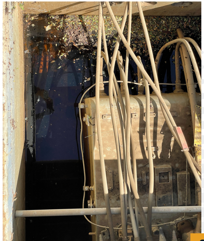
Underground utility enclosure holding water.
