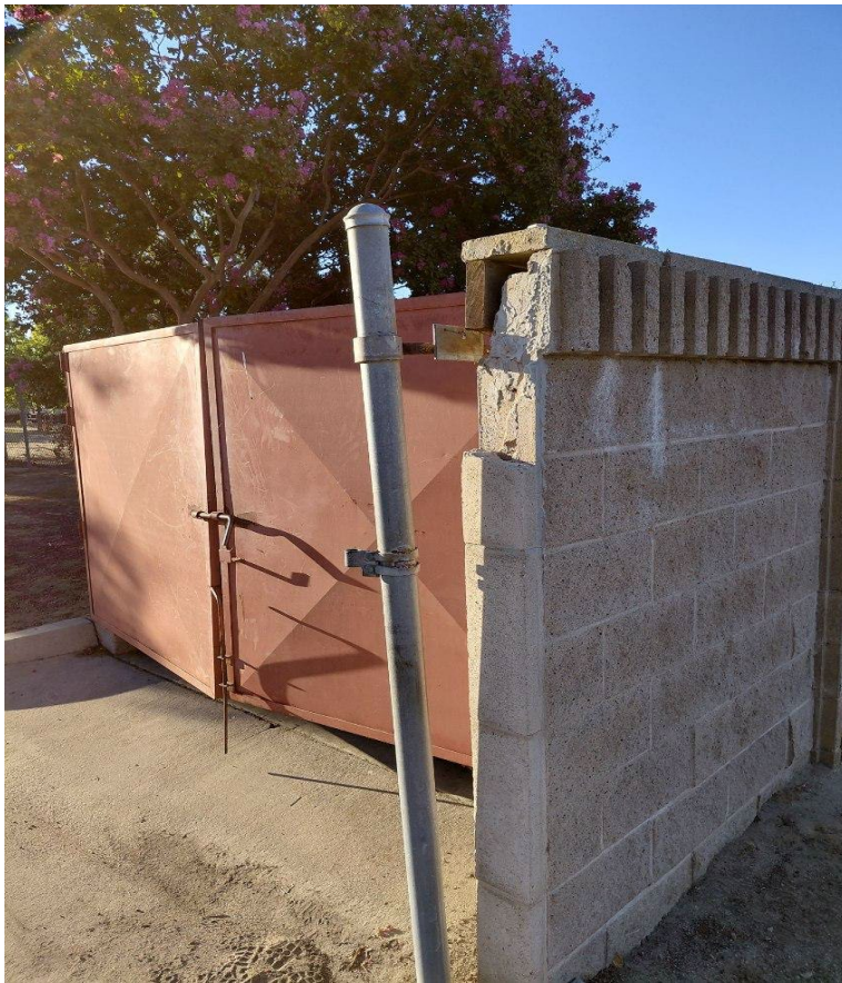
Cracked cinder block corner adjacent to the storage gate.
